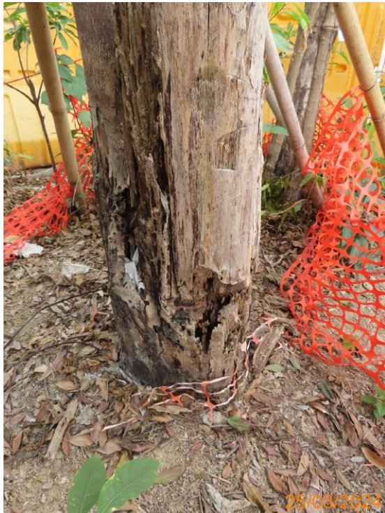
11: U041_Wood damage by termite
