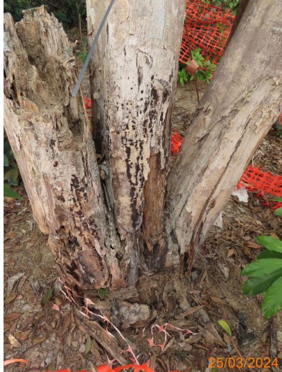
10: U041_Wood damage at trunk union
